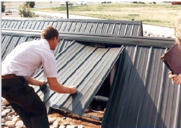
Figure G-6. Equipment Housing
